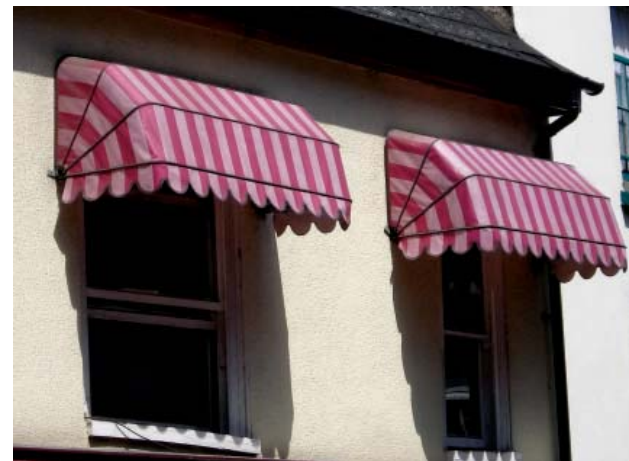
Dutch blinds are generally not acceptable
