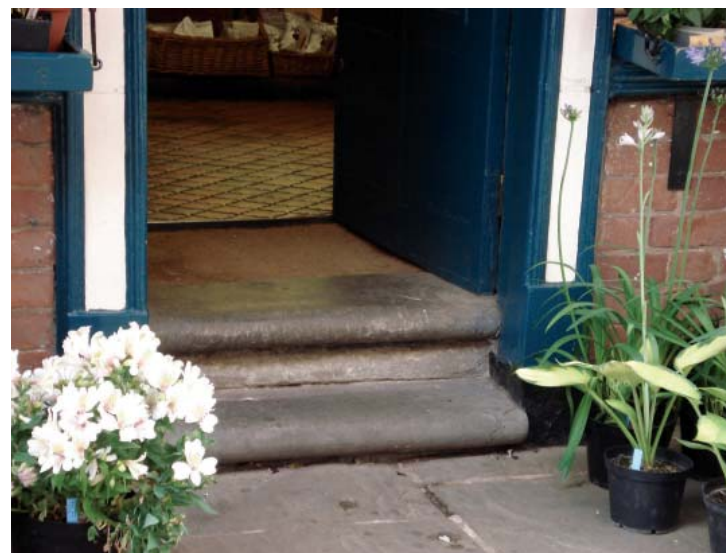
Rounded stone steps - part of the character of listed buildings. Difficult access for some customers
