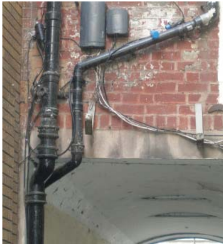
Untidy wiring and electrical boxes
